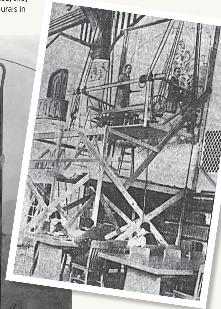
Above: Overmyer (right) and Wolfe (left) using scaffolding and materials supplied by K-State.
