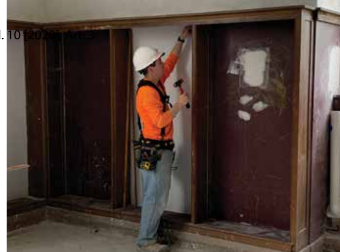
The original bookshelves located in the east and west alcoves of the Great Room are in the process of being restored. After the bookshelves are repaired, they are stripped and then varnished by hand.
