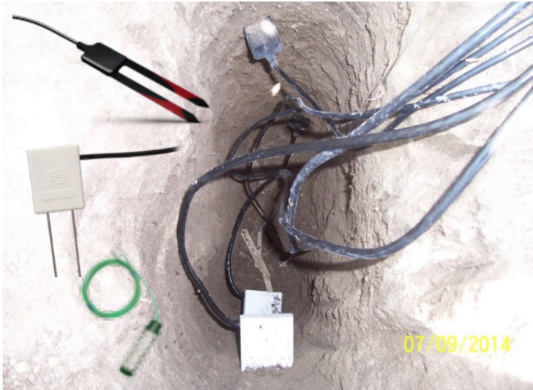
Figure 3. Three different soil moisture sensors (Watermark, CS655, and Decagon 10HS) installed at different depths (1, 2, and 3 feet) were established in the SWREC plot and a farmer's field.
